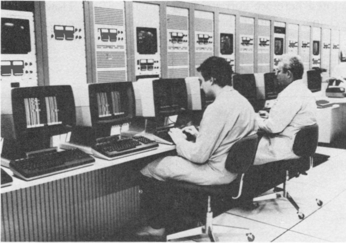
FIGURE 7.4 RCA Global Communications Computer Center. (Photo courtesy of RCA Globalcom.)
